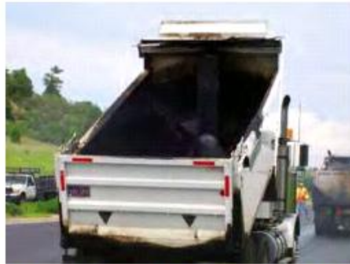
Once heated TBTRA is combined with the aggregate, it is hauled to the application site in tandem dump trucks (shown here).
